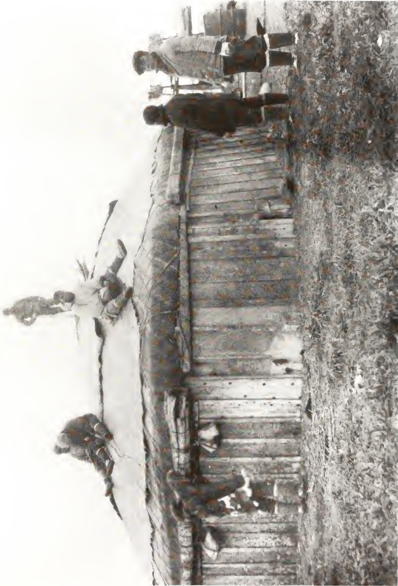
Gambell men (Waarmquun, Atalluk, Uveketaaq, Yughqutaq, and others) repair family winter house, 1912.
