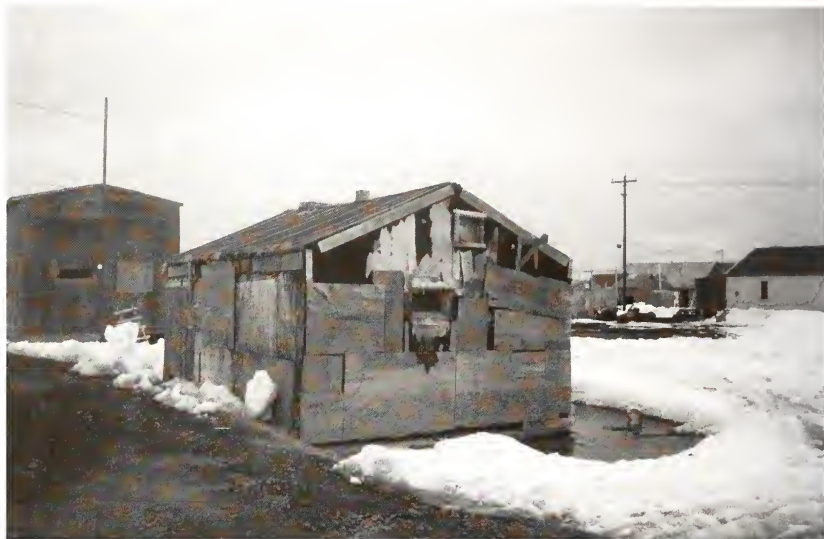
The old house of Piluwuk —the earliest remaining wooden structure of the “old town Savoonga,” 1999. Photographer, Igor Krupnik.
