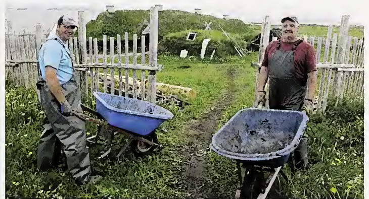
Fig 4.08: Workers rebuilding LAM had the advantage of wheel-barrows, a distinct improvement over hand-barrows 1,000 years ago. But otherwise, the scene and tasks would have been identical. Hand-barrows are still used in the northern fishing industry today.
