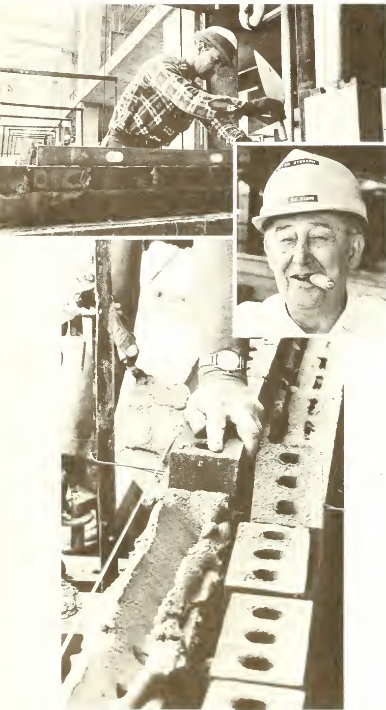
83-year-old Guy Kuhn, a journeyman member, Local 1, of the Bricklayers, Masons & Plasterers since 1911, demonstrates "laying brick to the line" as co-worker "butters the joints." Photo by Lou Hollis
