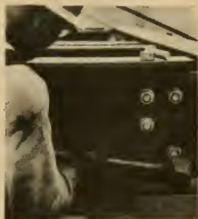
Beams that have been erected on previous days must still be set. First, the beam is "plumbed up" by two men with a hoist. In the next two pictures two "bolter ups" fasten the beam securely with bolts. Although bolts
