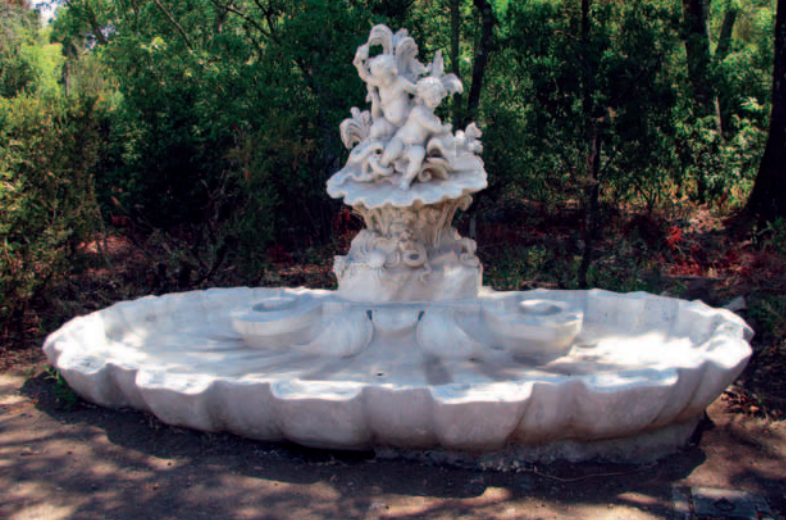
Fig. 7. Small shell-like fountain showing the problem of soil erosion under it (▲), and the Neptune fountain with extensive cracking in the bottom of the basin from roots of nearby trees.
