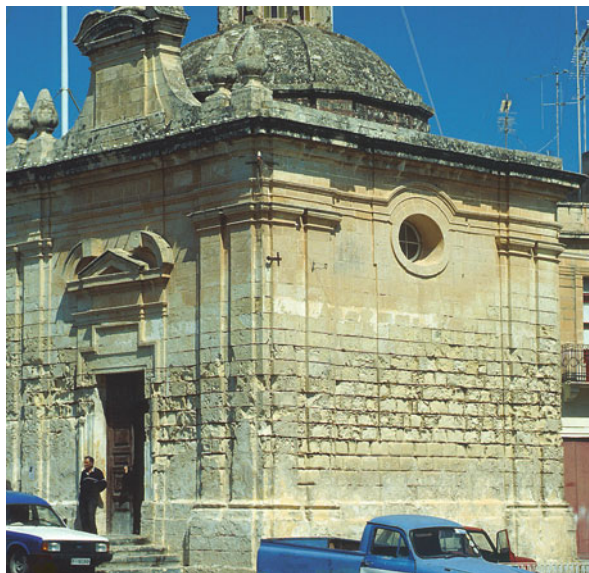
Fig. 4.17 Sea salt induced deterioration at Santa Marija Ta' Cwerra church (Malta); Photo: B. Fitzner, Geological Institute, RWTH Aachen University
