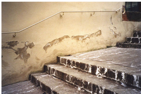
Fig. 4.18 Efflorescences of deicing salt on a stairway in downtown Basel. Reproduced with permission from Siedel (2009)
