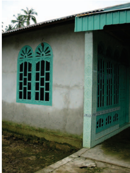
Figure 5. Water mark on house on Pulau Baleh; mark represents the daily height of water inundation at high tide. This house is approximately 70 m inland.
