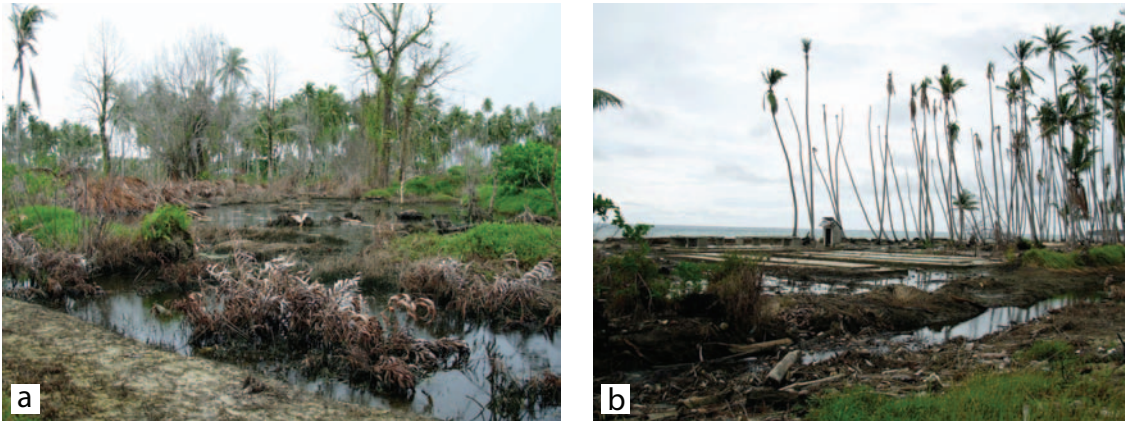
Figure 4. Terrestrial tsunami damage at Pulau Baleh showing (a) dead vegetation along the coast and (b) foundations of buildings that have been washed away by the tsunami wave.
