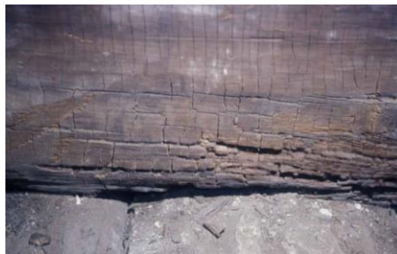
Soft rot in wallboard from the interior chamber of the King Midas Tomb
