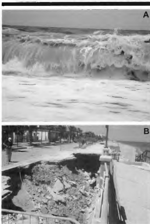
Figure 11. (A) Photograph taken in February 2006 showing normally strong winter waves breaking onshore and eroding the shoreface along Kaulonia's coastline. (B) Walkway (promenade) built in 2003 in Monasterace Marina, just south of Kaulonia, heavily damaged by storm wave surge effects in winter 2003–2004. In distance, note normally calm summer sea state at coast (photo: June 2004).
