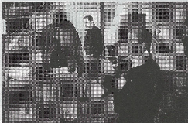
SI Secretary Michael Heyman hears Jana Harcharek outline the construction of the new Inupiat Culture Center in May 1997.
