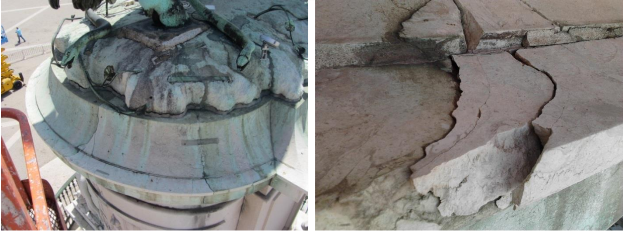
Figure 4. Details of the top and upper part of the plinth showing some fractures. Some of them were stabilised with bronze rivets during previous interventions (left). Detail of the fracturing pattern (right).
