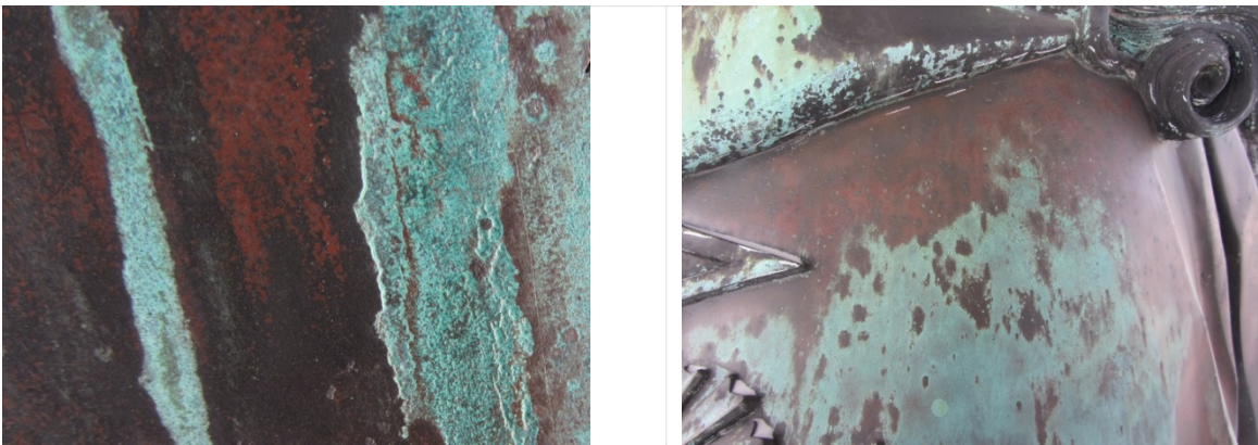
Figure 5. Aspects of the cuprite covered situation (coloured reddish) and its transition to the copper green compounds. Left: Cuprite is the underlying layer of the black soiling; the green stripes have formed along the water runoff paths and stay at a lower topographic level showing that erosion has already taken most of the cuprite layer. Right: During a cleaning test the black soiling was removed leaving an almost continuous cuprite layer. The green compounds encroach on the cuprite layer leaving behind some residual cuprite islands.
