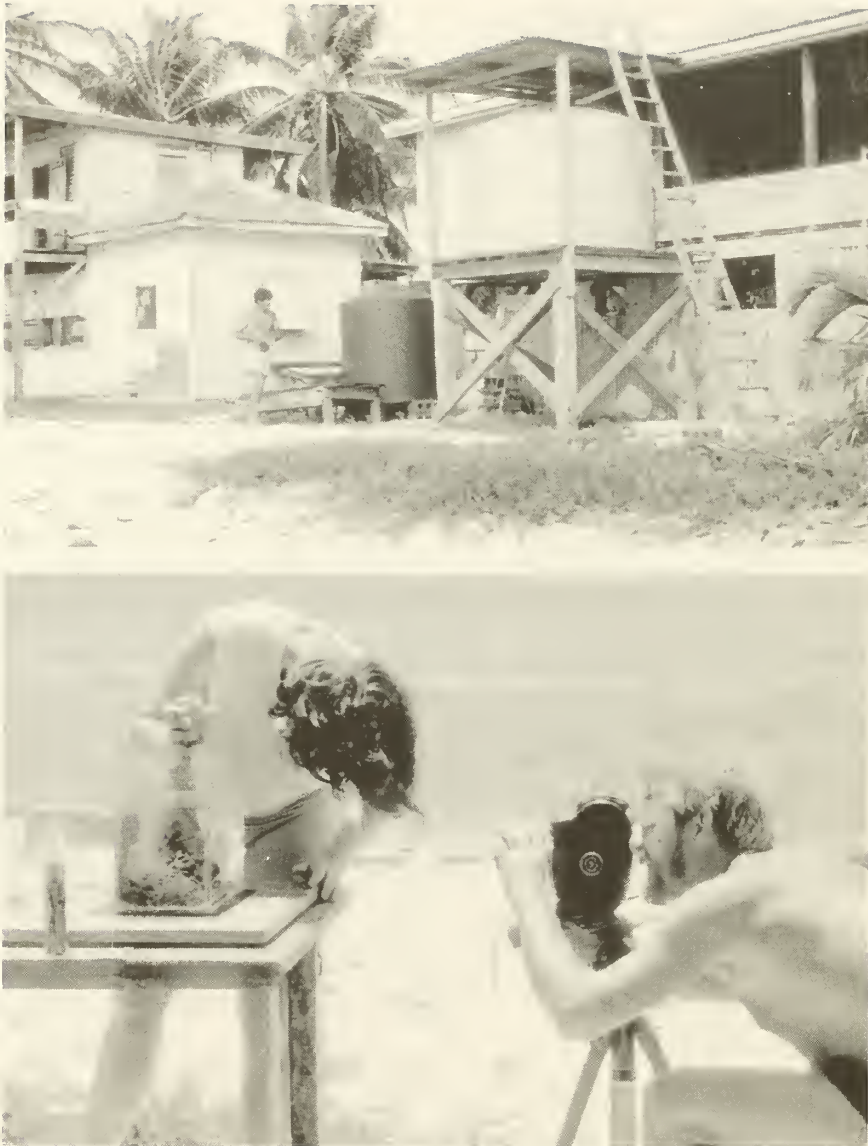
Figure 10. Renovating the Carrie Bow Marine Field Station with funds from the new CCRE Program (1987); Operations Manager Mike Carpenter is installing a large storage tank for the seawater flow-through system (top). Research assistant Kathleen Smith positioning sponges for filming water-pumping activity made visible by fluorescent dye (bottom).
