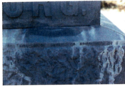
Fig. 7. Lowville, NY, monument showing a typical white-bronze base, with damage from inappropriate repair by filling it with concrete (since removed). Conservation Solutions, Inc.
