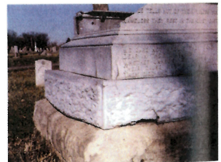
Fig. 3. Zinc plinth of Confederate Monument, Bardstown, KY, showing cracking and deformation from metal creep. Note rustication on zinc intended to match stone base. Conservation Solutions, Inc.
