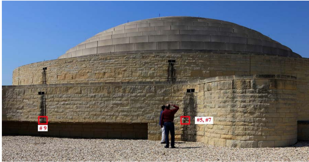
Figure 2. Left, view of the east face of the 5 th floor terrace showing locations of samples #5, #7, and #9 from darkened areas below two scuppers, which drain water from the small terrace above and, in turn, the main roof terrace with the dome (April 2010).
