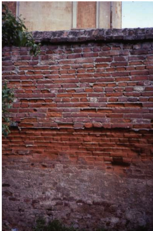
Figure 9: Old brick masonry wall in a garden that was repointed with a cement mortar. Note that major damage occurs in the center area where salts crystallize out as subflorescence (between half a meter to 1 m height) and that the bricks are damaged first being more porous than the cement mortar. The lower area, where the wall is mostly damp, concretions tend to form with salt efflorescence right above it, but less damage is evident.
