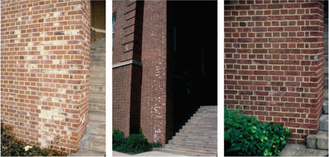
Figure 3: Detail of the brick masonry at the portal (Figure 2 right) on the left side as it appears in winter (which are dry, T < 3^{\circ}\text{C} , RH \sim 50\% ; left) when efflorescence is most visible; in spring (where humidity increases, T \sim 10^{\circ}\text{C} , RH between 60 and 85%; center), and during summer (which are damp, T \sim 30^{\circ}\text{C} , RH between 70 and 90%; right) where practically no efflorescence is visible because of the hygroscopicity of the sodium sulfate. The salt is inherent to the brick and mainly crystallizes out near the edge of the arch where more evaporation takes place.
