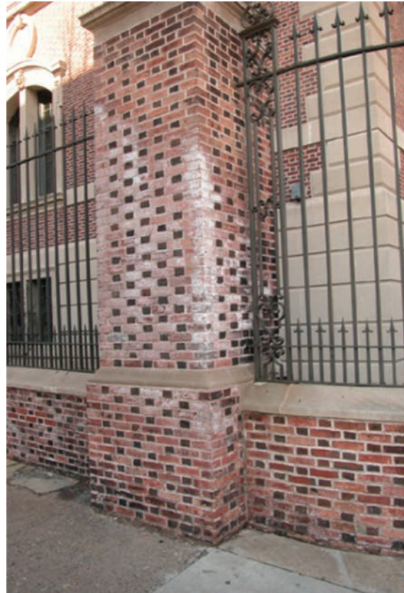
Figure 4: On the fence surrounding the Silverman Hall Law Building of the University of Pennsylvania, efflorescence began to appear one year after its cleaning (1999) and continued to increase with each passing year. While the cleaning products were properly washed off from the building itself where no salt deterioration occurred, this careful procedure was not applied for the fence (Photo January 2005). Efflorescences are visible during the dry winters, while in the humid summers, these areas appear damp.
