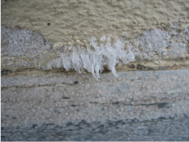
Figure 6: The paint of a façade is detached by the growth of long salt whiskers (over 1-cm long) that mechanically push away the paint from the surface.
