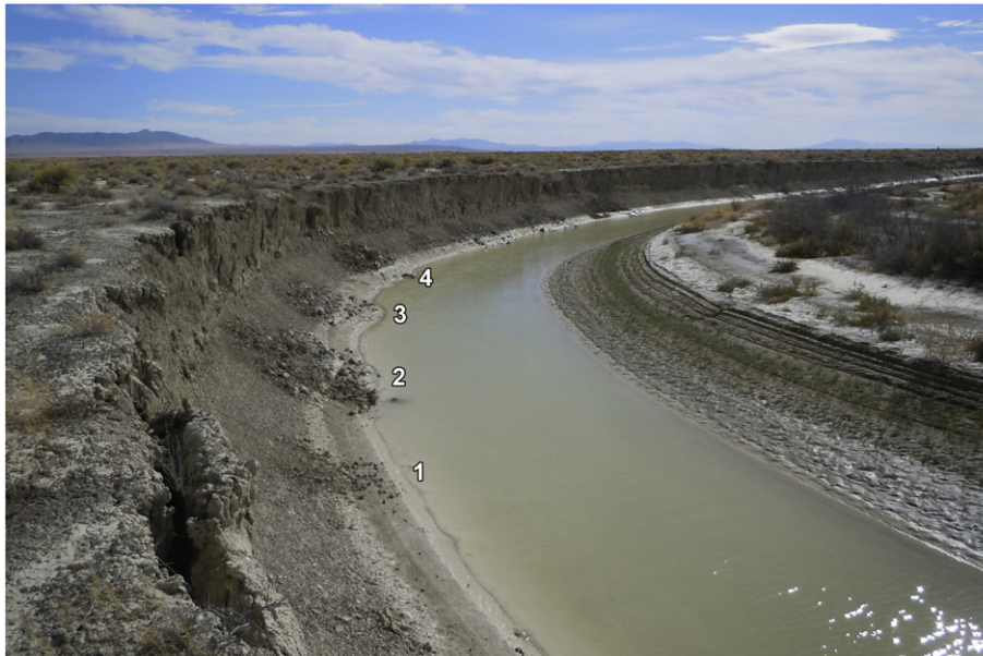
Fig. 17. Mass wasting and fluvial features along a meander bend of the Quinn River, looking downstream. At this location the channel is eroding into Lake Lahontan sediments. Bank height on outer bank is 3.6 m and on the inner bank is 2.1 m. The right bank shows a typical expression of inner bank sediment deposited by oblique accretion. Short scarps on this bank reflect notching of bank during water level decline, presumably by wave action. The spring, 2011 high water was just above the highest notching and within the light-toned band with scattered low shrubs. Line of shrubby vegetation along the crest of the right bank marks an older scroll bar. The silty sand deposits comprising scroll bars are conducive to vegetation growth. Note that the prominent water mark on the left bank is well below the level of the 2011 high water, which probably reached to the break in slope on the bank. Mass wasting of small blocks from the steep upper bank has mantled the high water bank textures. A recessional water stage on the left bank is indicated by damp, light-toned smooth bank extending about 0.6 m above the present water level upper banks fail by block by block or by cantilever failure along tension cracks. Note incipient failure in foreground and numbered debris fans. Bank failure 4 occurred prior to the recessional level and its deposits below that level have been extensively reworked with the exception of a few partially eroded blocks at water level. Bank failure 3 may have occurred during the recessional water level and is partially reworked. Note that the disaggregation of the debris has produced a convexity in the bank at water level. Bank failure 2 may have had two separate events, being partially smoothed below the recessional water mark but with angular debris deposited after the water level had retreated to its present value. Bank failure 1 occurred after the recessional water level but while the river level was several centimeters above its present level. Image located at 41.192°N, 118.738°W and taken on October 15, 2011.
