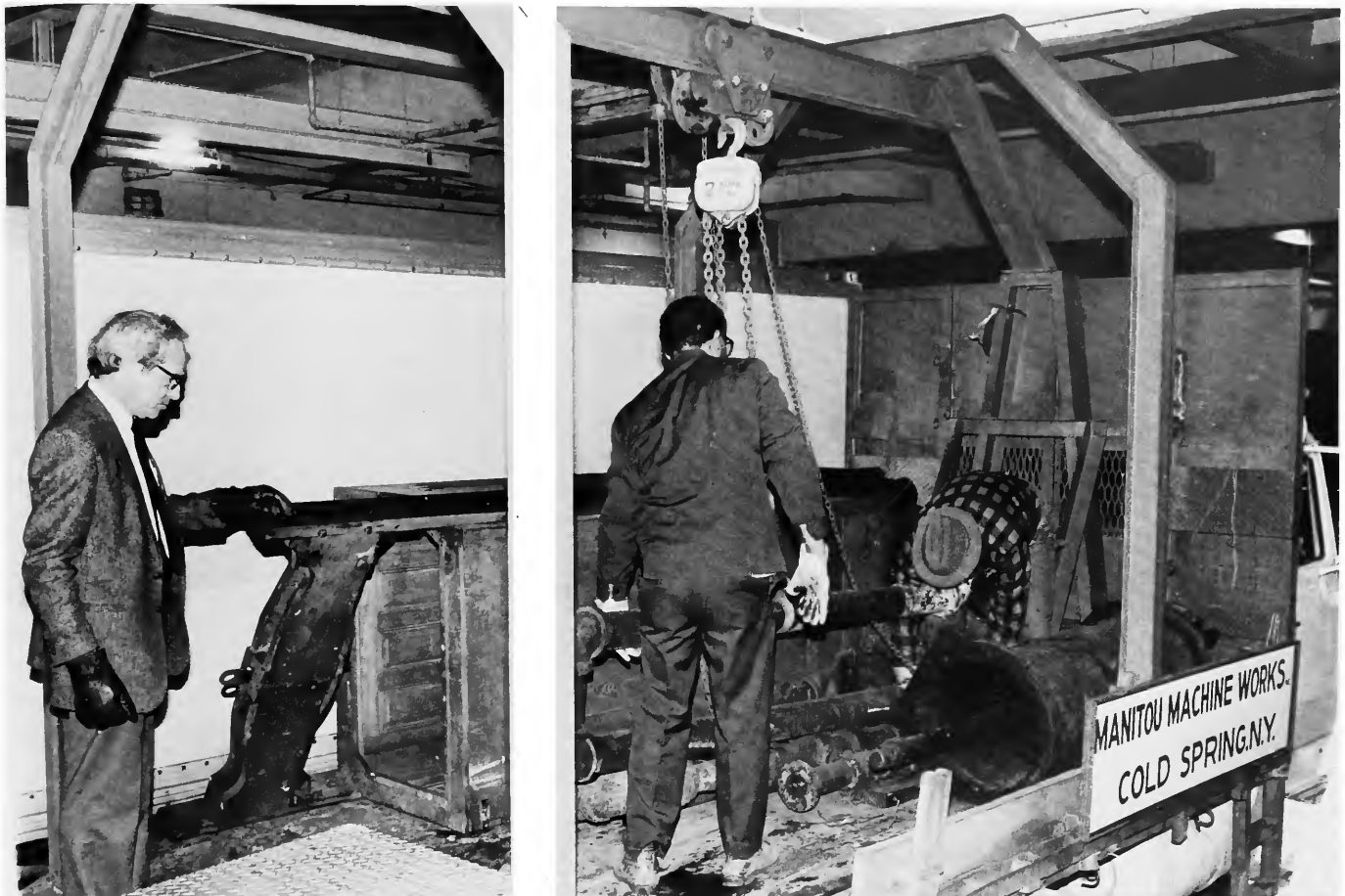
FIGURE 18.—Arrival of the elevator at the National Museum of American History, “knocked-down.”
