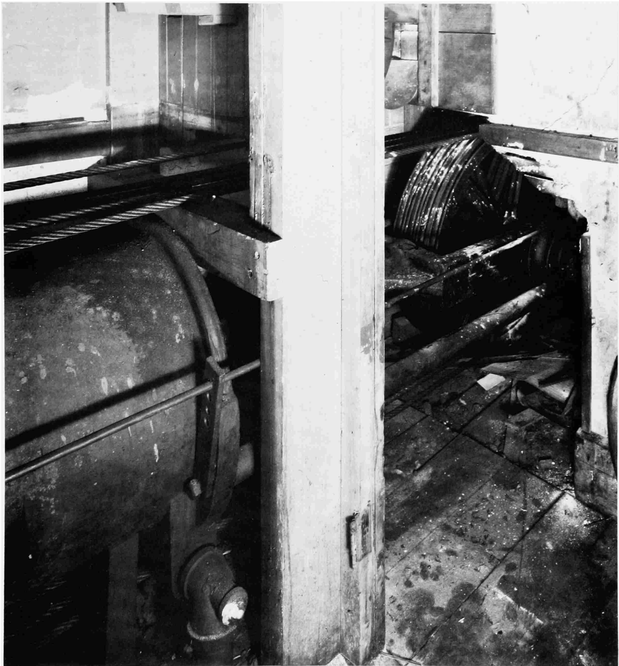
FIGURE 14.—The traveling sheaves and their inner guide rail, tucked neatly beneath the bottom run of the basement stairs. (Jet Lowe.)
