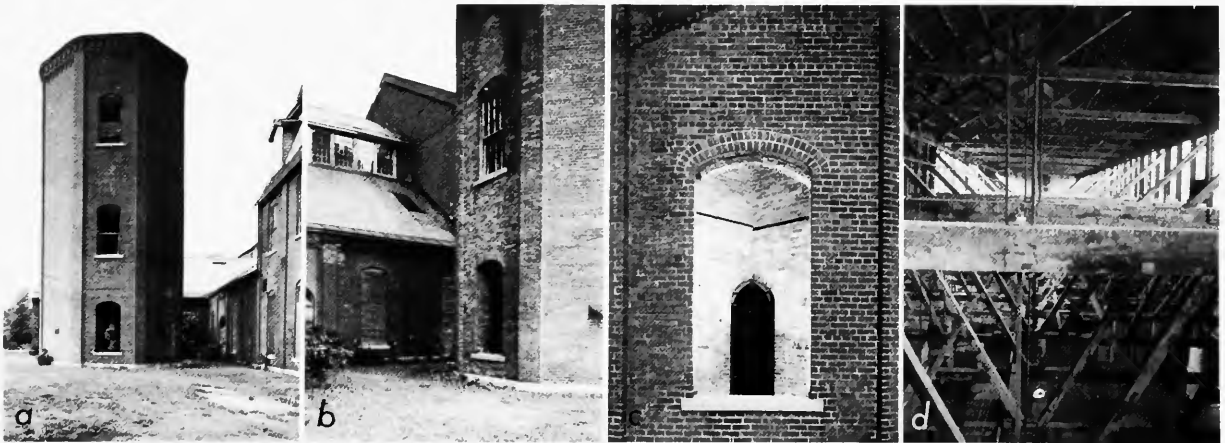
FIGURE 140.—Green Island Shops: a , Brick water tower base; b , joining of machine and locomotive shops and north face of water tower base; c , window in water tower base, showing diaphragm walls that supported tank floor; d , interior of the north section. ( a-c : Boucher; d : John Courtney Fisher for [N.Y. State] Division for Historic Preservation.)
