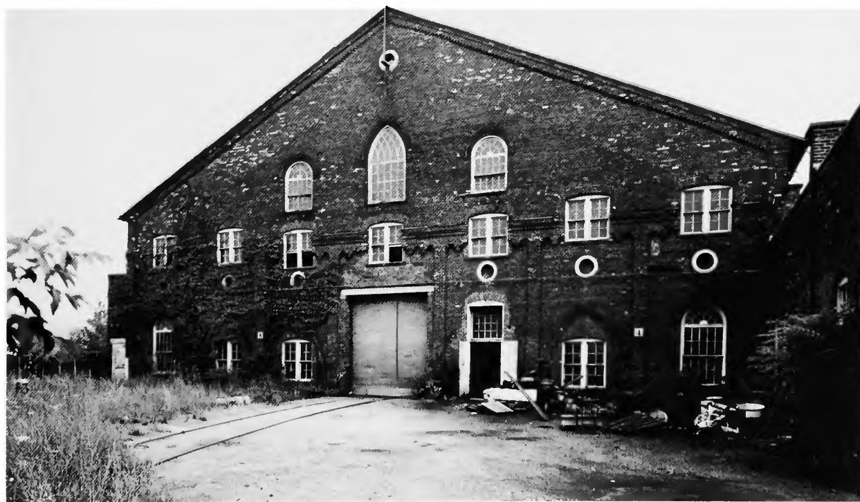
FIGURE 42.—North elevation of Rail Mill showing outline of the original monitor roof in the gable end.
