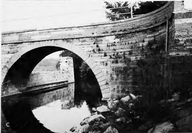
FIGURE 128.—Upper Mohawk River Aqueduct: a , West face of the aqueduct at the south bank of the Mohawk; b , view from the southeast of the piers that supported the timber trunk; c , view from the southwest showing the canal trunk bed and the south abutment; d , towpath arches from the southwest.
