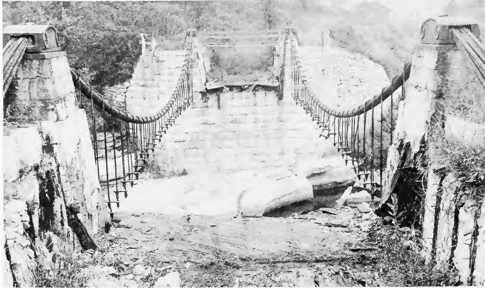
FIGURE 108.—After standing derelict for nearly twenty years following abandonment of the canal, fire destroyed the wooden trunk of Roebling's Delaware & Hudson aqueduct at High Falls, New York, c1916. The cables and suspenders were left in a state not unlike that during original construction, just before the first of the trunk frames had been hoisted into place. (Courtesy of Delaware & Hudson Canal Historical Society, Gear Collection.)
