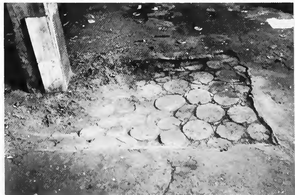
FIGURE 44.—Rail Mill, section of floor of northeast corner of building. Log sections, of undetermined length, probably were employed as an inexpensive and relatively durable surfacing, anticipating (or imitating) commercially produced end-grain-block industrial flooring; or perhaps what is seen here are the ends of a cluster of close-driven pilings that formed the foundation for a heavy machine.
