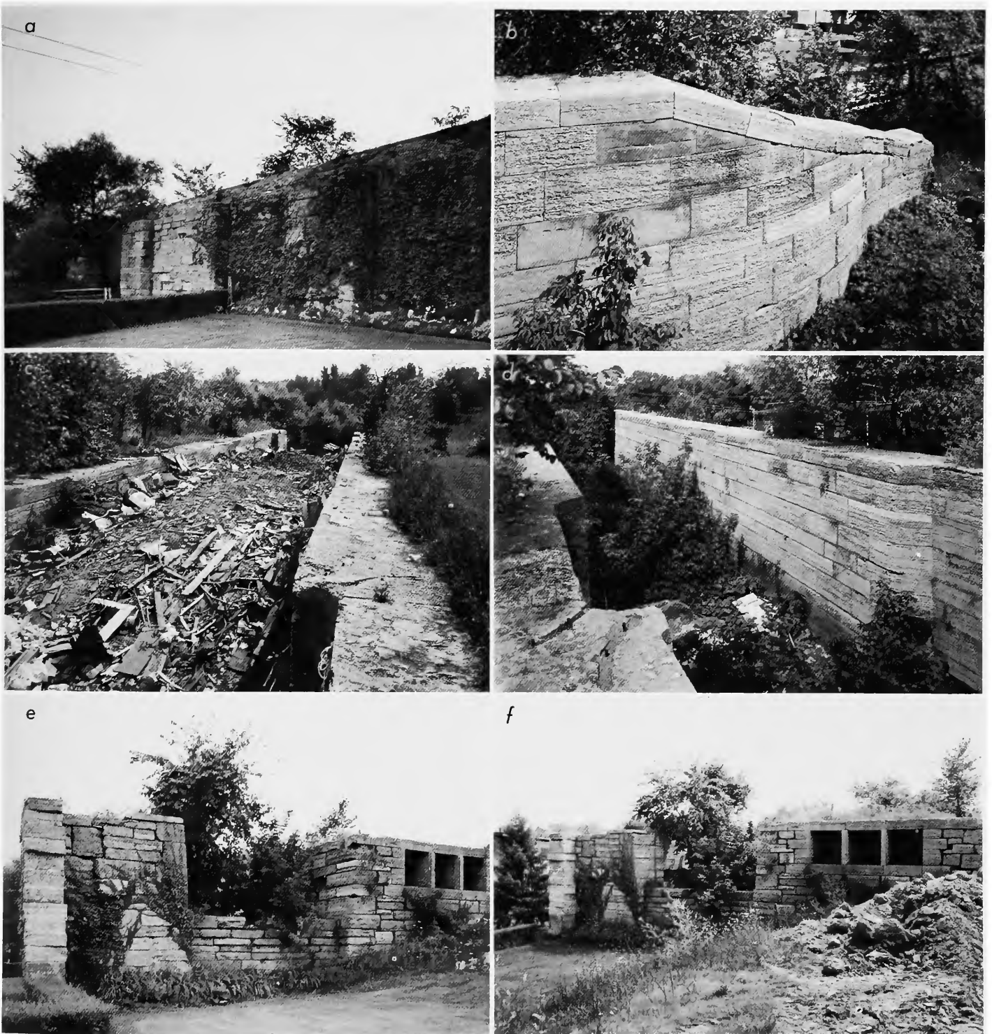
FIGURE 130.—Lock 18: a , East face of lock structure; b , foot of wall at southeast corner of Lock; c , east lock chamber, looking south; d , east chamber, looking northeast; e , north (upper) face of lock, showing filling ports; f , north face.
