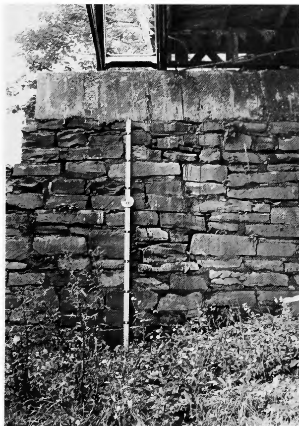
FIGURE 7.—Field photograph (35 mm) with measuring pole placed against the structure, another method of increasing recording efficiency (abutment face, Whipple Bridge).
