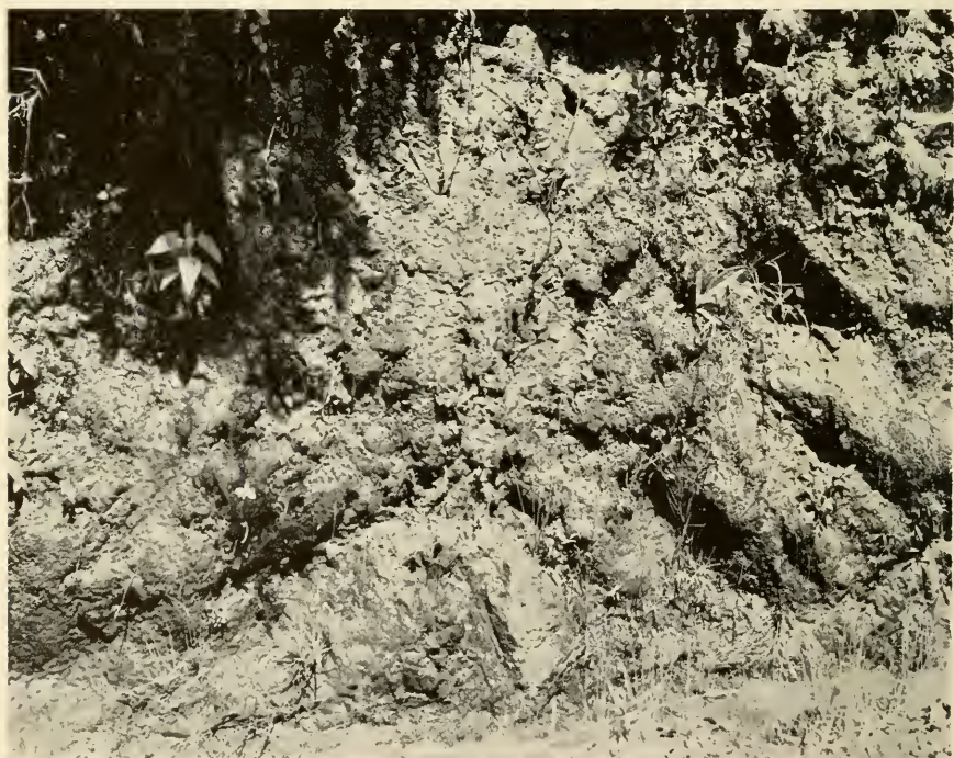
2. Seepage from large area of wet-faced wall, from which streams originate.
