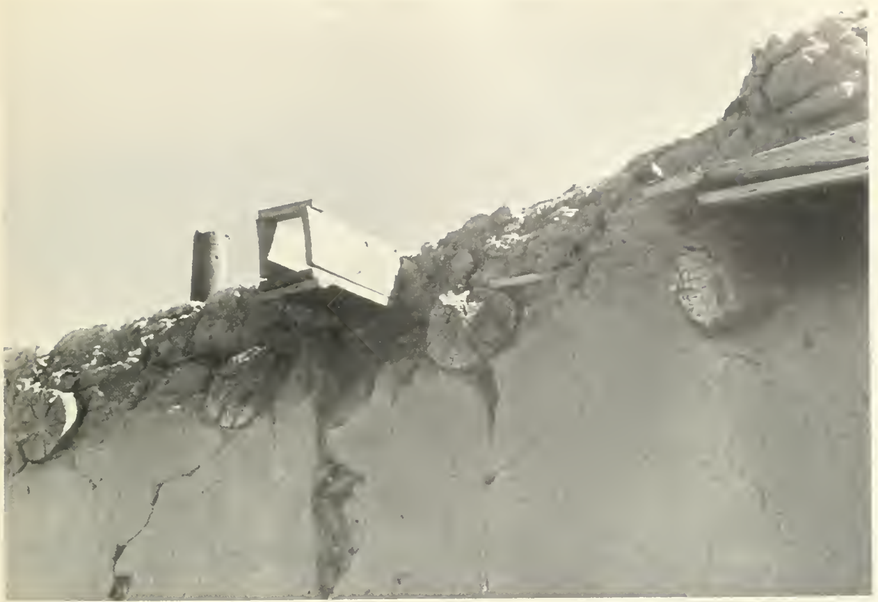
FIGURE 3. North roofline of east morada , showing exposed ends of ceiling beams ( vigas ), chimney of oratory stove, and construction of water drain ( canal ).
