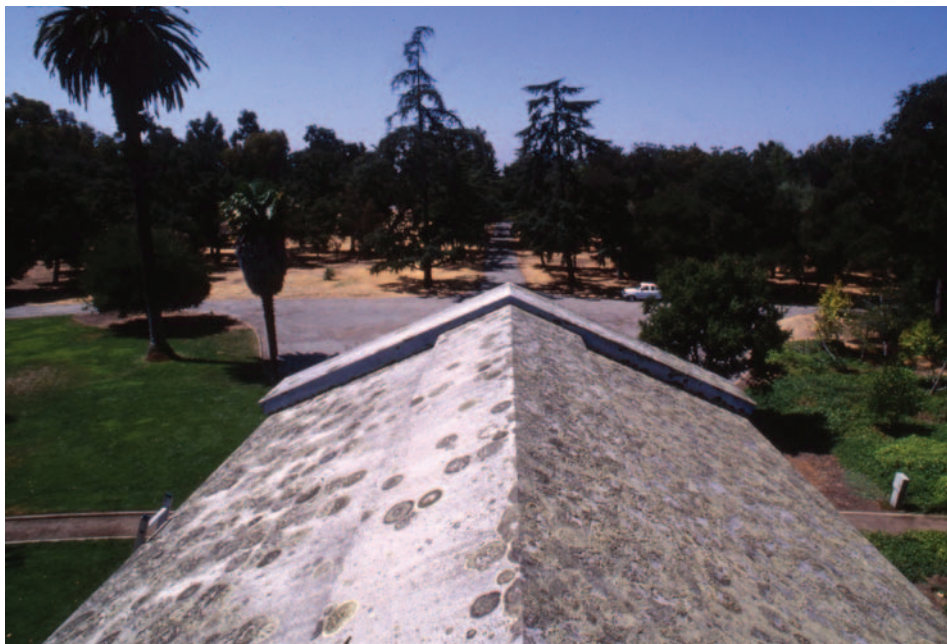
FIGURE 2. The roof of the Stanford Mausoleum in 1995, showing the heavy lichen colonization that had developed over 106 years.
