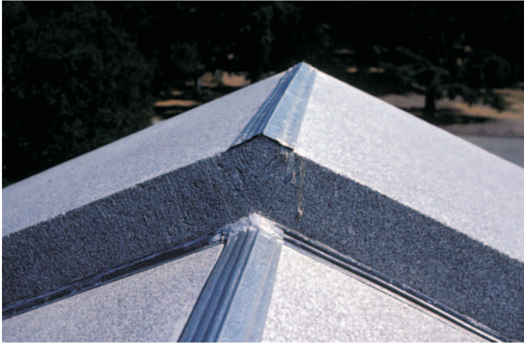
FIGURE 3. The roof of the Stanford Mausoleum after cleaning in 1997, showing the zinc strips installed on the roof's ridges.
