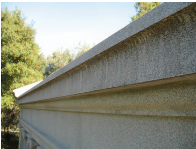
FIGURE 6. Detail of the cornice in 2009, showing new soiling.
