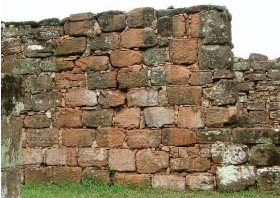
FIGURE 6. View of the side of the wall three months after hand removal of higher plants and brushing on all test areas (photo taken December 2008).
