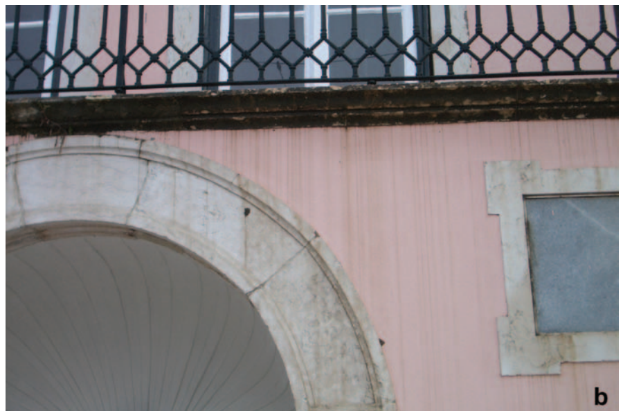
FIGURE 5. (a) Detail of a limestone sculpture treated with a water repellent, showing the resulting streaked pattern where biocolonization develops (Villa Pisani, Stra, Italy). (b) Detail of the garden wall of the Palace of Belem (the residence of the president of Portugal) in Lisbon. Note that only the render is water repellent, showing the streaking effect. On nonhydrophobized surfaces, such as the stone in the arch and around the plaque, colonization is more diffuse.
