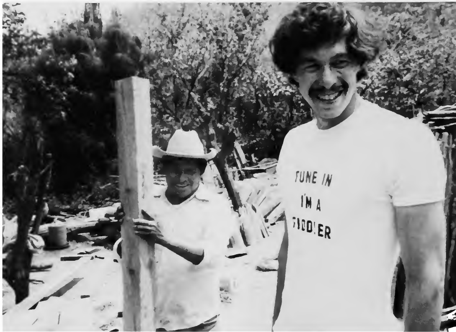
FIGURE 23.—The fiddler, John B. Haviland, with Romin Peres Peres, rebuilding the roof of his dream house in Naben Chauk, 1984. (Photo by Frank Cancian.)
