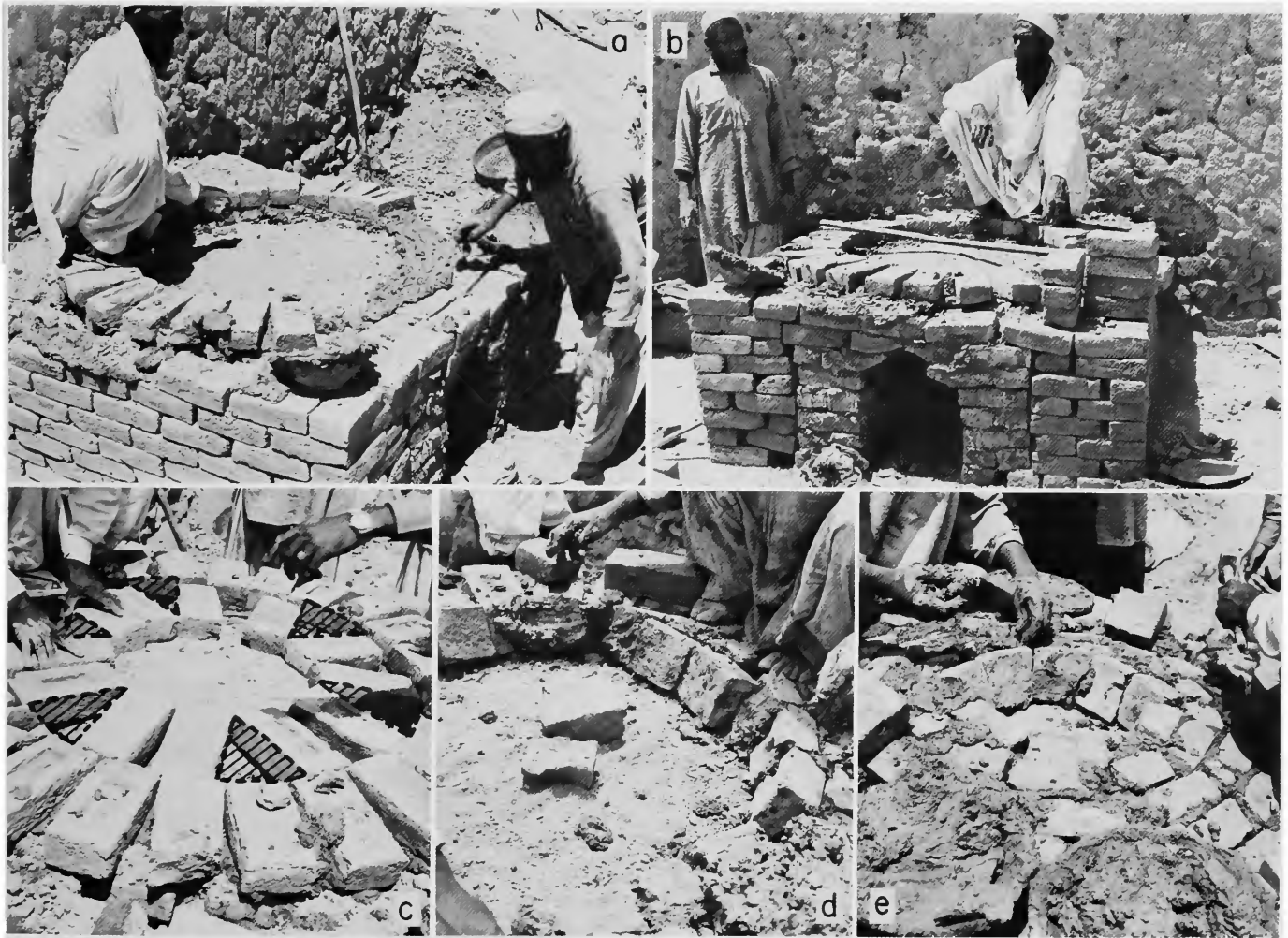
PLATE 64.—Potter Roshan Din demonstrating kiln construction, Zakhel Bala, NWFP (continued): a , wood/clay formwork completed, a further radial course of bricks laid; b , ready to build the domed floor, rise of the clay formwork for floor may be compared with stick placed across top; c , using bricks to measure off equidistant spaces, and determine position of flamethroats (broken lines); bricks are removed after location of flamethroats has been determined; d , e , commencing floor construction (bricks laid in circular pitched (on edge) courses). (See Plate 65.)
