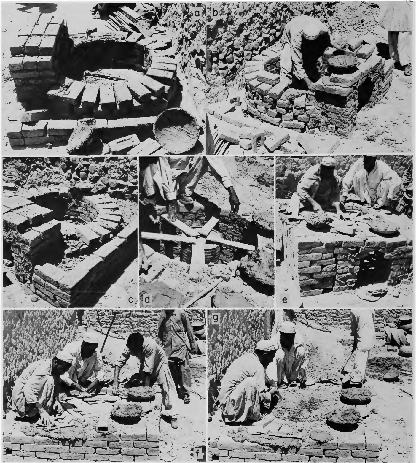
PLATE 63.—Potter Roshan Din demonstrating kiln construction, Zakhel Bala, NWFP (continued): a , firebox (circular) completed up to fourth course (note radial course); b , continuing construction of firebox; c , outer insulating wall completed to fourth course (gap between firebox and outer wall filled with dry clay); d , building a chamber floor, a steel drum used to support wooden formwork; e , f , wooden formwork to support floor is placed in position; g , formwork covered with dry clay, level with brickwork at edges and raised in center. (See Plate 64).
