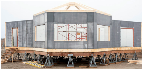
Top: Kuugalak's Elder design committee overseeing the unloading of construction materials. Bottom: The Kuugalak workshop under construction. Photo by Margaret Thompson Photography
