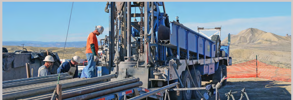
(Below) USGS core drilling rig for assessment of natural gas in the Mancos shale formation (USGS)
