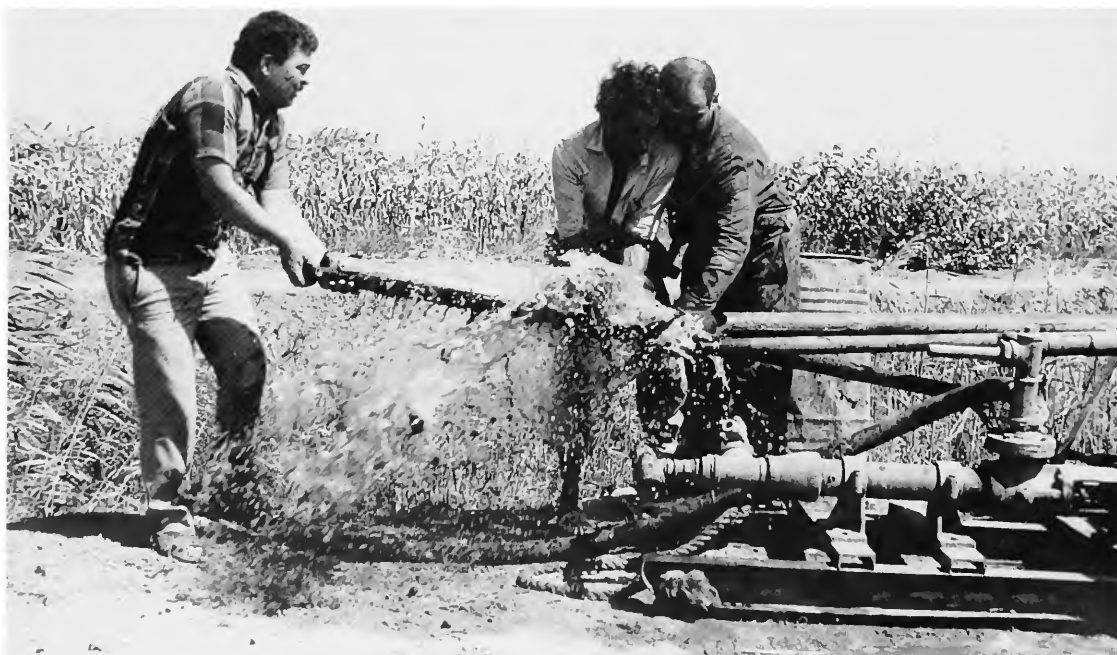
FIGURE 4.—Extrusion from drill pipe of stiff clayey silt of late Pleistocene age, using high pressure pumping of circulated water. Photograph taken at site S55 in September 1989.
