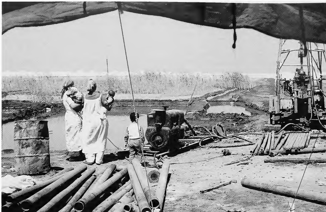
FIGURE 3.—Large-diameter pipes in foreground are used for casing, particularly when drilling in thick sections of sand and/or soft mud. Note 10-foot (3.05 m) lengths of drill pipe assembled near the drilling equipment. Photograph taken at site S11 in September 1985.
