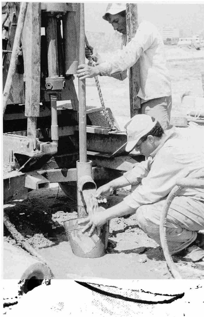
FIGURE 5.—Recovery of sediment from washings of circulated water in a thick sand sequence. Photograph taken at site S77 in September 1990.
