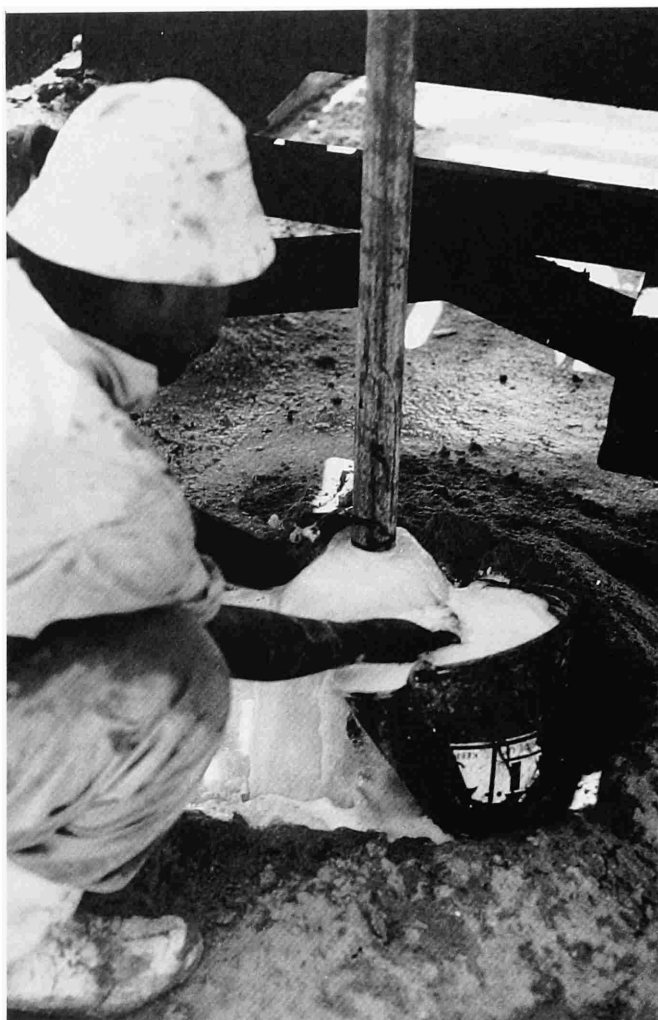
FIGURE 6.—Drilling through consolidated carbonate section of late Pleistocene age in the region west of Alexandria. Pumped water is typically white when circulated through drilled carbonate sequences. Photograph taken at site S85 in September 1990.
