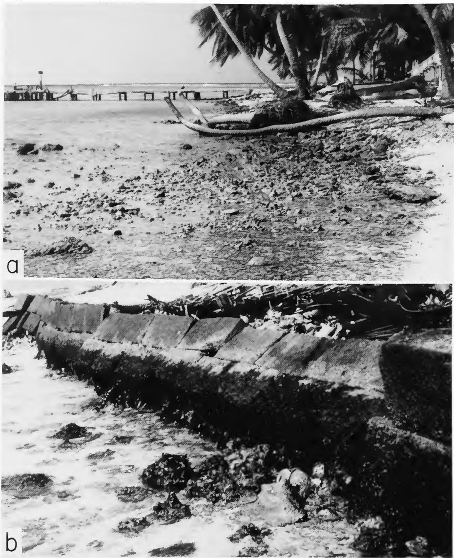
FIGURE 52.—Intertidal substrates: a , sand and rubble (mainly conch shells) on western shore, looking north (coconut palms felled by hurricane Greta); b , northwest seawall, coated by algae Cladophoropsis and Oscillatoria , topped by Greta .
