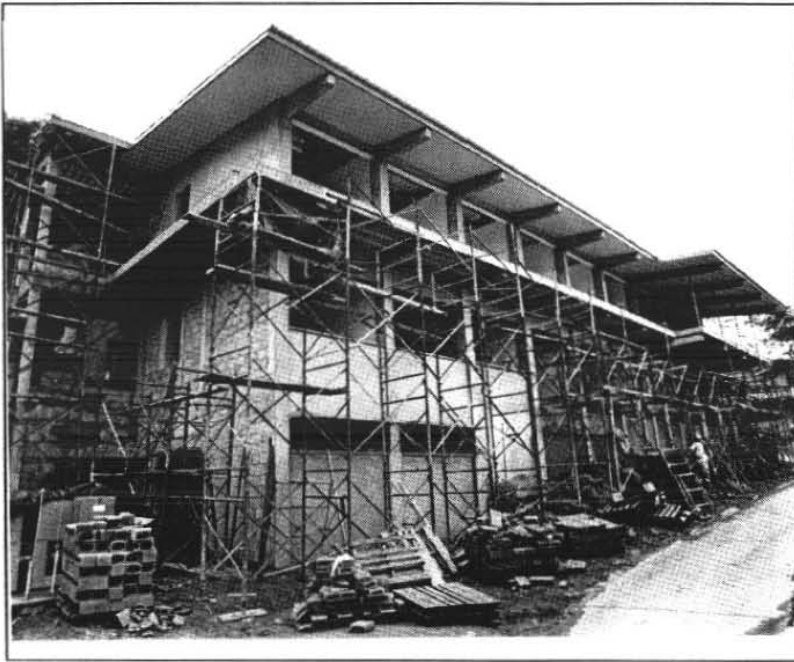
Construction of laboratories, dormitories, pier and a special storage facility at BCI is scheduled to be completed in October. The photo shows the south wing of the laboratory building. (Foto: M.A. Guerra)
