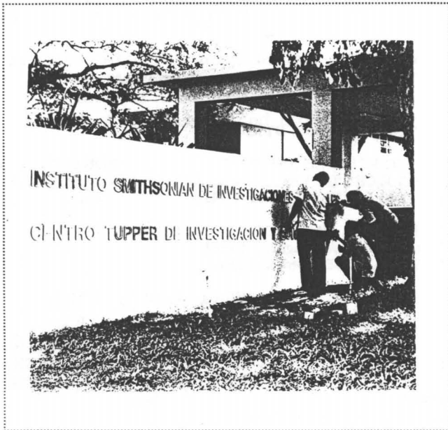
Construction workers from Don Ted S.A. are seen installing the new sign identifying the Tupper Center. (Photo by M. Guerra)
