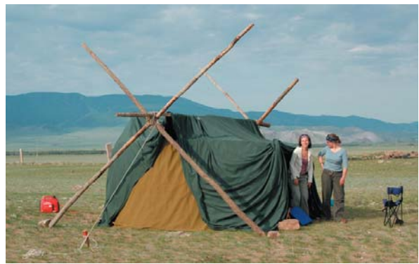
Fig. 20 The completed ger shade shelter for deer stone #3 at Ushkiin Uver (June 2006)
