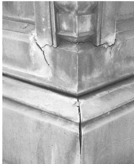
Fig. 9. Detail of a corner of Nevada's Tribute to Union Soldiers and Sailors (1891), showing cracks resulting from concrete filling, white bronze, Lone Mountain Cemetery, Carson City, Nev. Photograph by Carol A. Grissom
