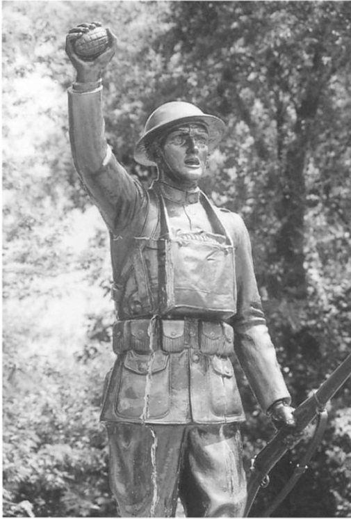
Fig. 10. E. M. Viquesney's Spirit of the American Doughboy (1944) showing cracks resulting from plasterlike filling, bronze paint on cast zinc, Verona, Pa. Photograph by Carol A. Grissom
