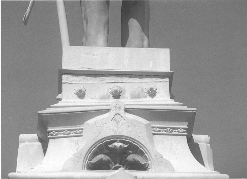
Fig. 7. Detail of fig. 6, showing the leveled statue and Pliacre fill just below its self-base. Photograph by Carol A. Grissom
