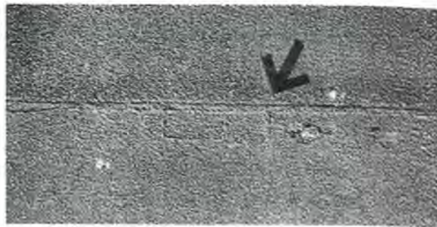
Figure 3. Original Aquia Creek sandstone repair (dutchman) at the center of the photograph, indicated by an arrow.
