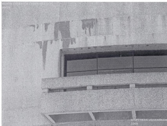
Figure 1. Condensed water leaking from the joints in the wall of the Smithsonian Institution's Hirshhorn Museum and Sculpture Garden in the wintertime. (Photo by Gary Johannsen and Kevin Guifreda)
