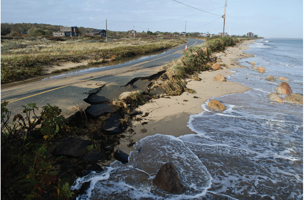
Figure 12. Damage from storm surge at Lobsterville Dunes following Hurricane Sandy, October 31, 2012 (A.O. Fisher).
