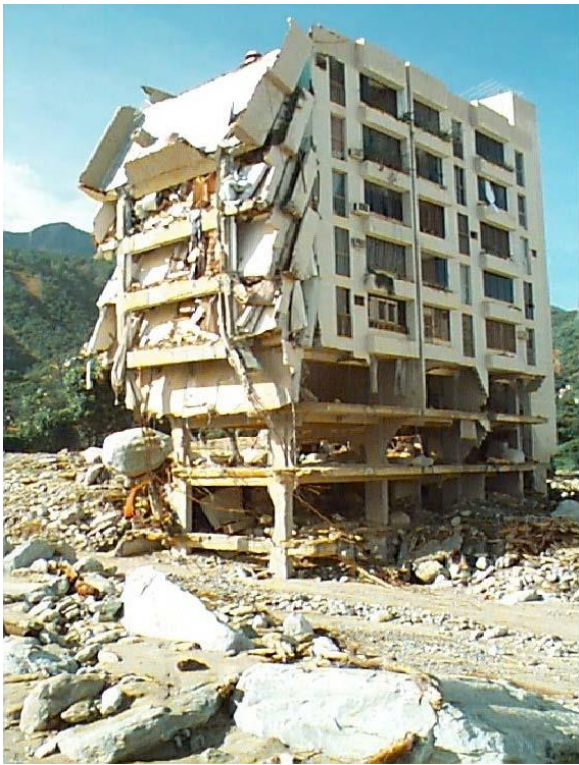
Figure 6. Apartment buildings damaged by debris flows and flash floods, 1999, Caraballeda, Vargas, Venezuela. Photo source: M.C. Larsen, January 2000.
