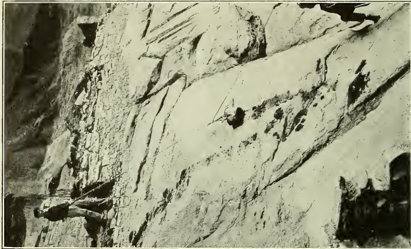
B. FOR REPAIRING THE EAST HOUSE GROUP, MUD WAS DRAGGED UP THE SLOPE FROM COURT 83
