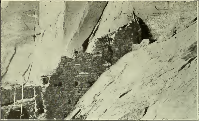
A. THE NORTHWEST WALL OF ROOMS 64-65 (WHICH LATER COLLAPSED) WITH BEAM HOLES MARKING THE FLOOR LEVEL OF THE SECOND-STORY CHAMBER
