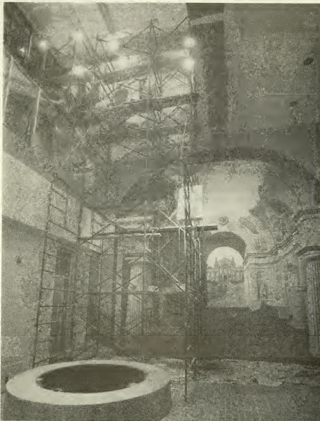
Viewed through scaffolding, an illusionist mural designed by artist Richard Haas nears completion underground in the Quadrangle building. The mural, providing a dramatic end to the building's monumental concourse, depicts the Castle (upper left) and the Arts and Industries Building through ancient stone arches. (Photo by Jeff Tinsley)
