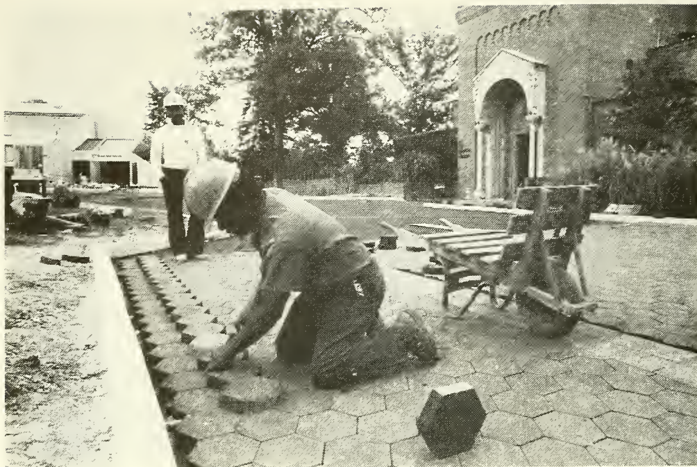
Workman lays hexagonal pavers along Olmsted Walk, the main pedestrian path through the National Zoo. The renovation of this walk should be complete by 1989, in time for the Zoo's centennial. Photo by Jessie Cohen.
