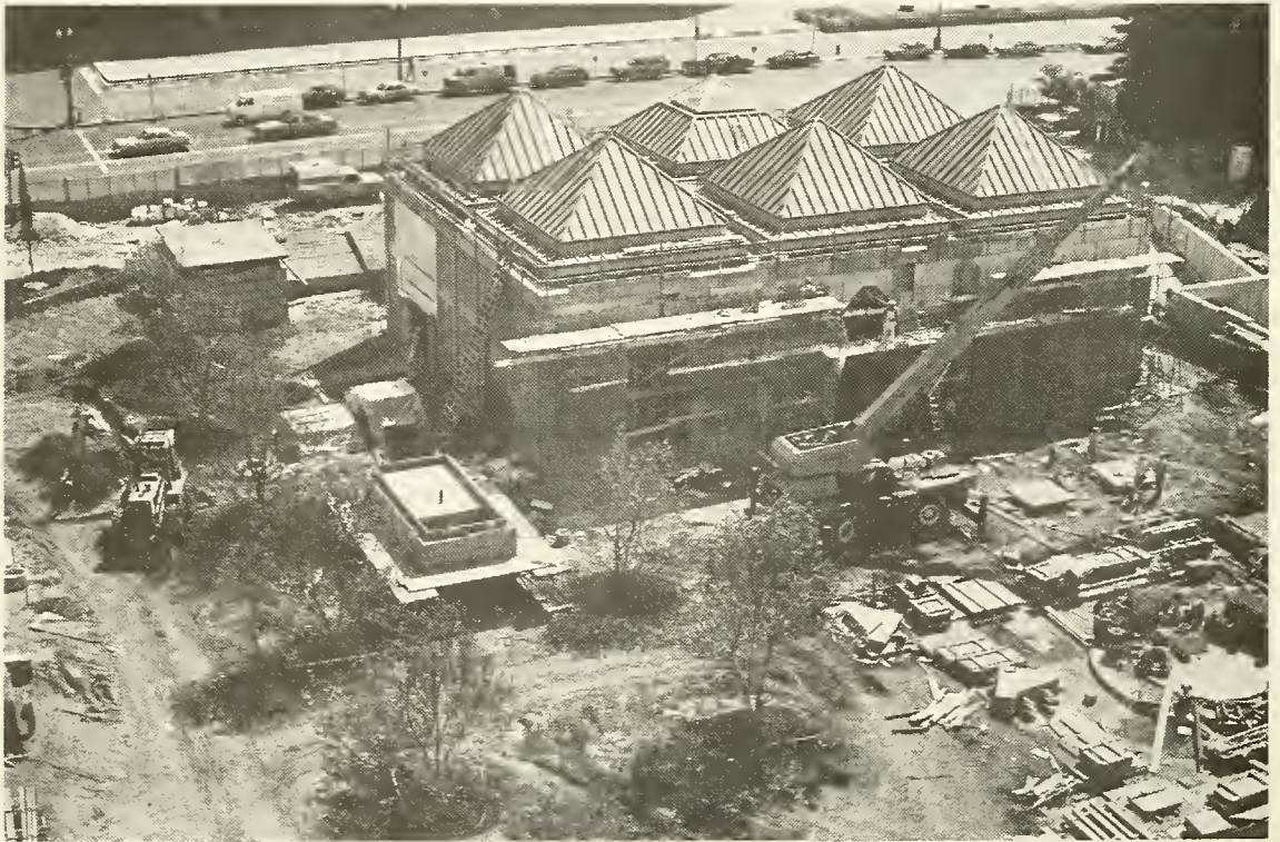
Quadrangle construction nears completion. Upper photo shows African pavilion copper roofing and skylight, with fountain construction in the foreground. Lower photo shows granite installation on Sackler pavilion north facade and completion of copper roofing. Photo by Frank Gilmore.
