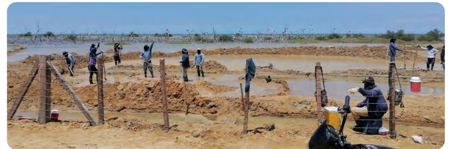
Local and ancestral knowledge informed the process of digging channels to secure water flows to and from the mangroves in Musichi. © Adriana Daza
